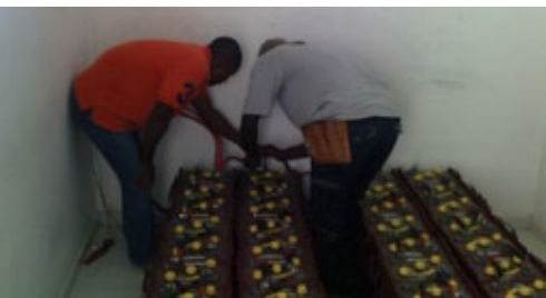
48 Trojan L16RE-2V batteries Photo by Jeff Korcan, courtesy of Solar Electric Light Fund
