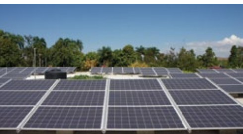
Thomonde hospital, Haiti Photo by Nadia Todres, courtesy of Solar Electric Light Fund
